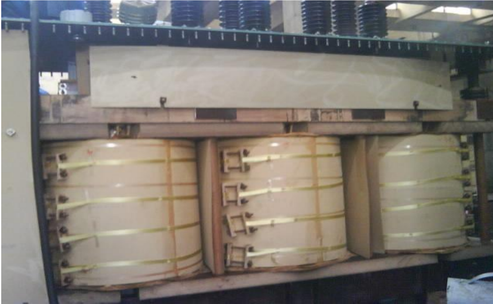
Winding of a 40-MVA ,66/11 kV transformer.
