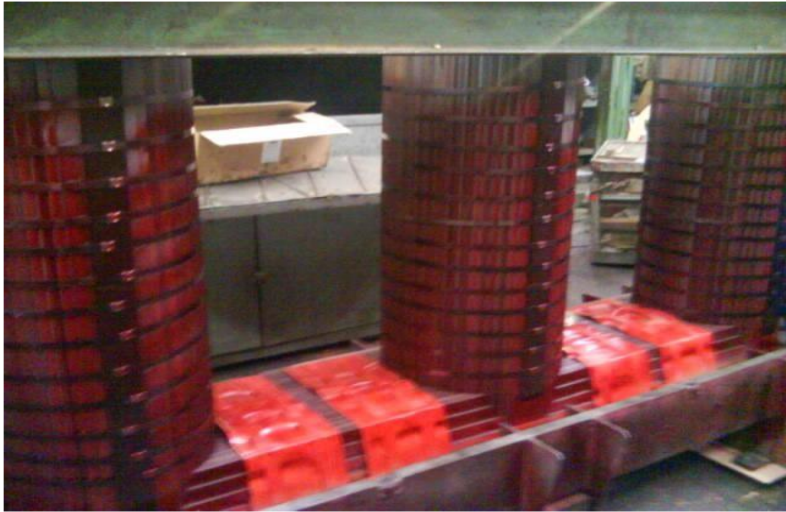
Core of a 40-MVA ,66/11 kV transformer
